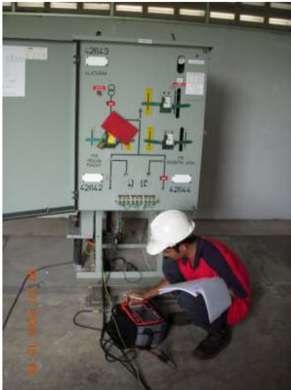
a) Offline testing set is connected with the earth connector must be connected to earth
